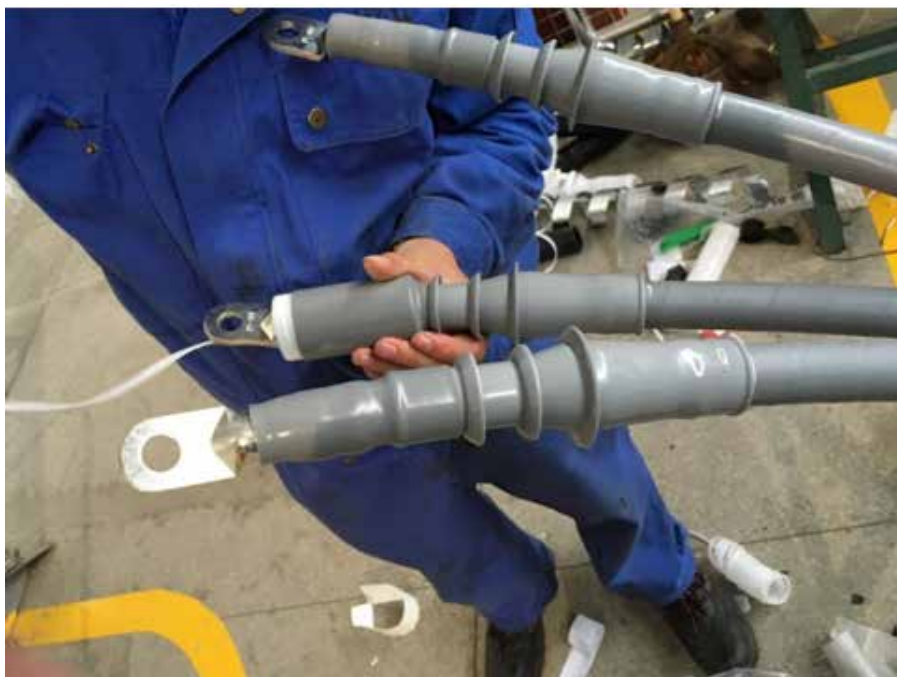
Today’s outdoor terminations are factory produced and tested. Source: Ivan Jovanovic, director of engineering specialty products with G&W Electric and associate member of PDI 2 .
