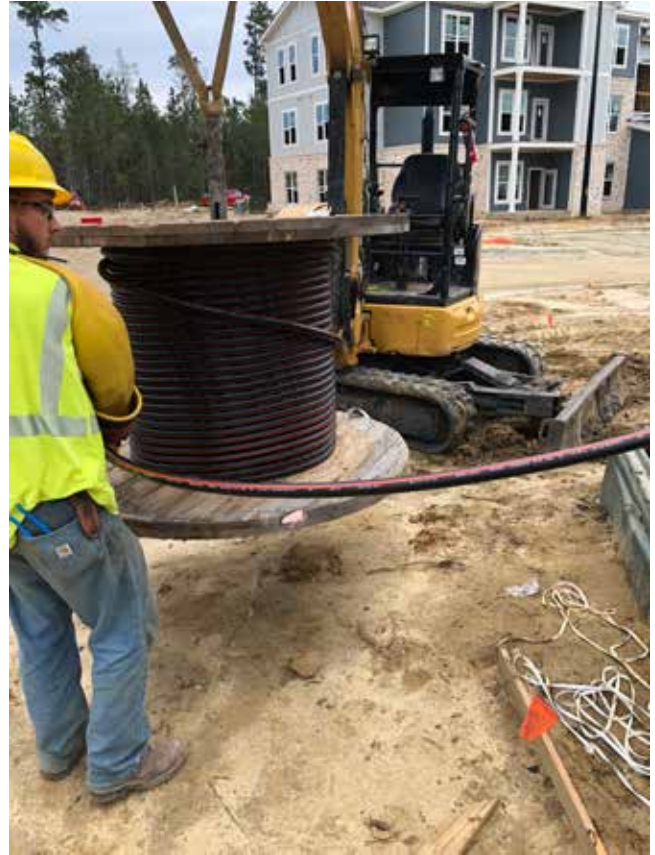
Low-cost cable installation in South Carolina. Source: Brian Hunter, regional manager of TT Technologies and associate member of PDI2.
